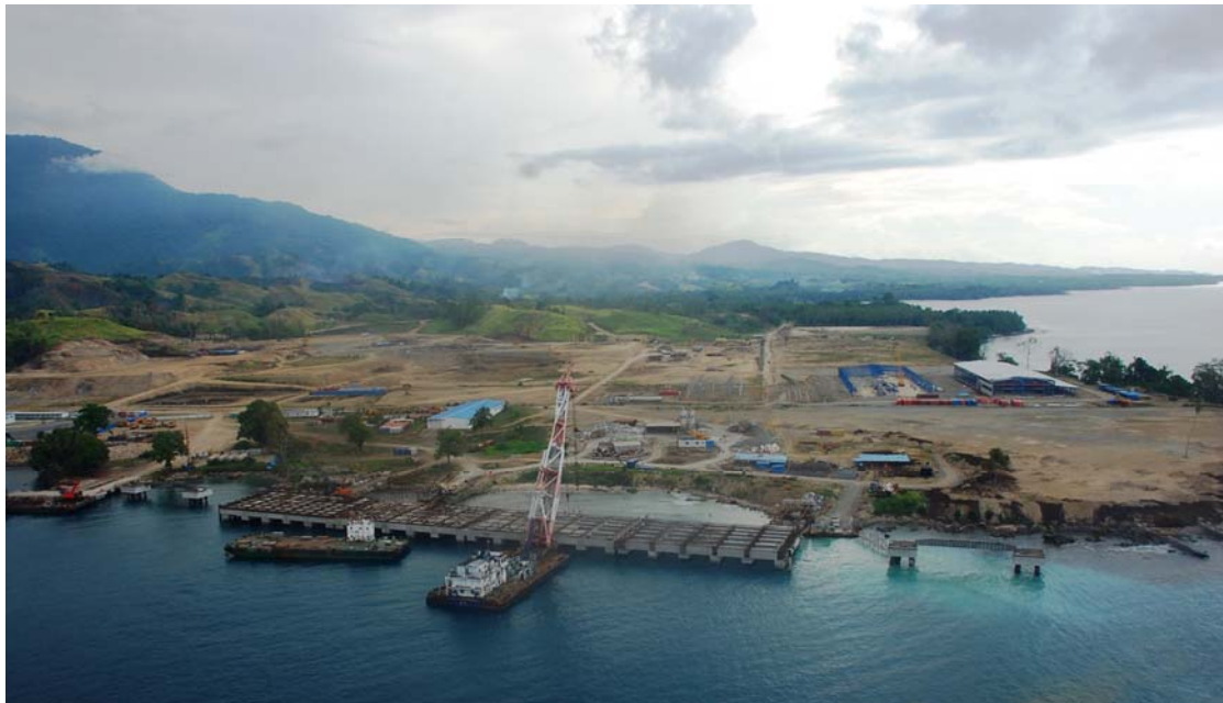
Construction of the Basamuk Wharf and Process Plant Area Ramu Nickel-Cobalt Mine
